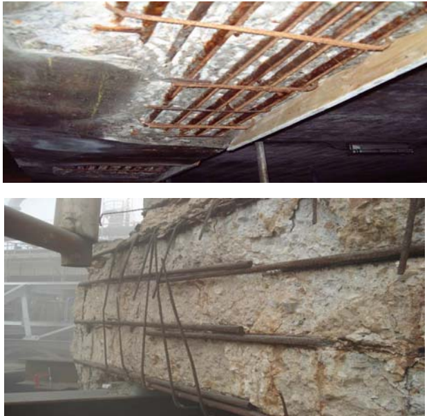
FIG. 1:- CORROSION IN BEAM
